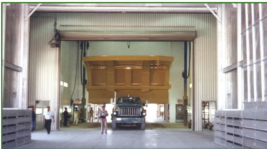
View of paint system building interior showing the part moving into the convection oven.
