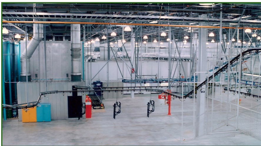
The completed powder coat line at Honda's Timmonsville, SC ATV manufacturing facility.
