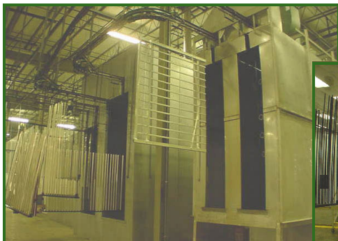
Exiting the 3-stage dual-pass pretreatment machine at Jerith Mfg. Co.'s facility in Philadelphia, PA.
